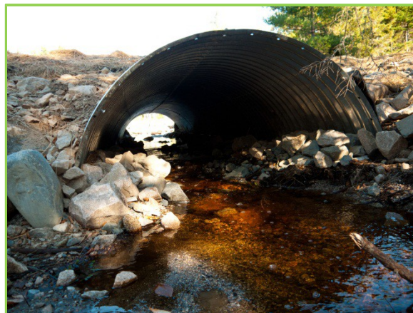
Figure 37: Black Rock Brook culvert looking from the downstream side. Photo by Nancy Sferra.
