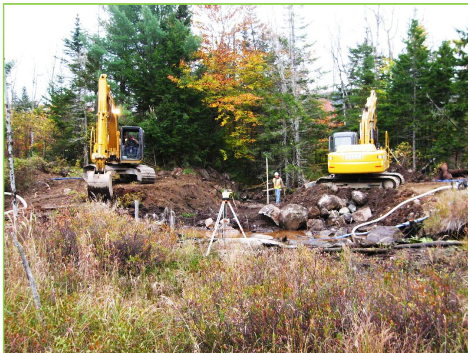
Figure 26: Construction work at Black Rock Brook site, October 2011. Photo by Dan Grenier.
