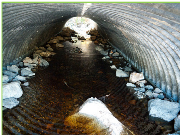
Figure 36: Black Rock Brook culvert looking from the upstream side. Photo by Nancy Sferra.
