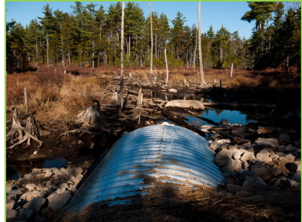
Figure 33: Black Rock Brook downstream following installation of new culvert. Photo by Nancy Sferra.
