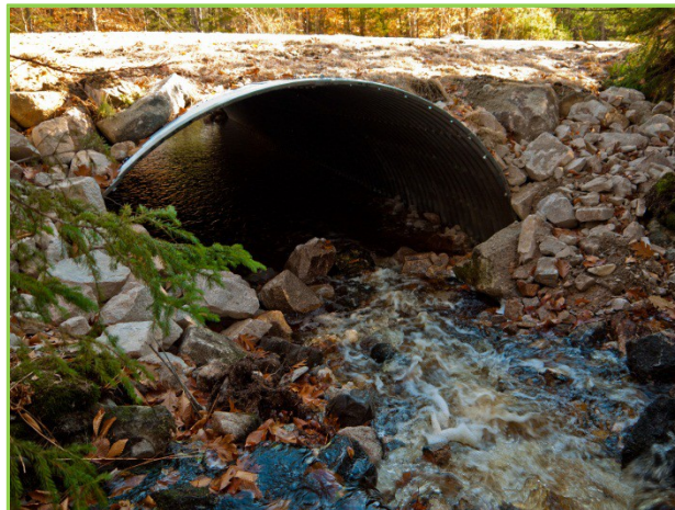
Figure 31: Ash Bog Stream upstream of culvert following installation of new culvert. Photo by Nancy Sferra.
